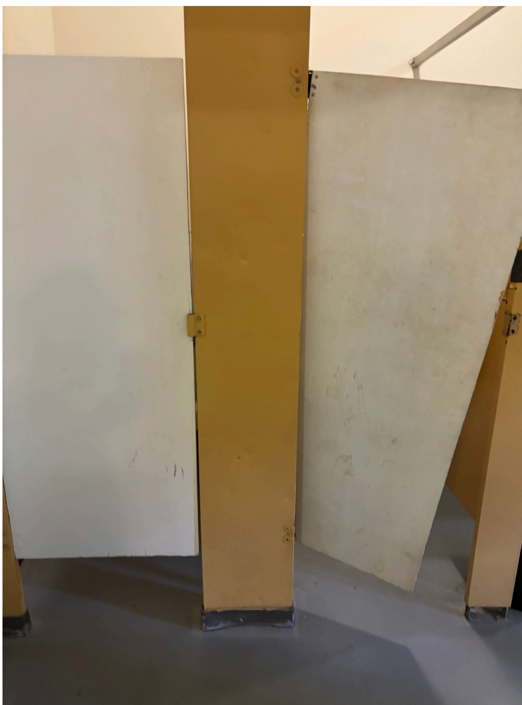
Broken boys’ sport locker room stalls - Chase Parkinson
