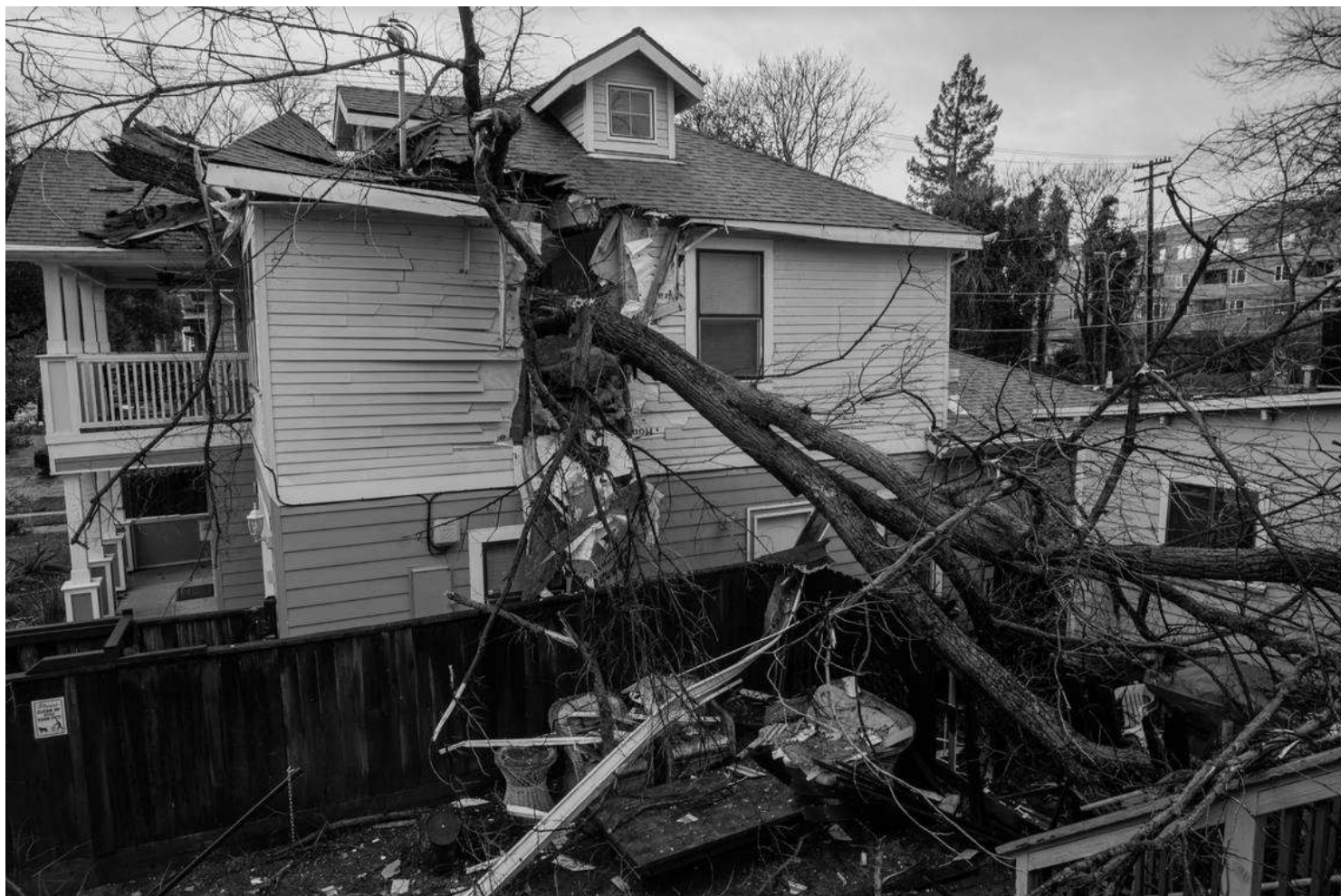
A fallen tree pierced through a home near 13th and D streets in Sacramento's Mansion Flats neighborhood on Wednesday, Jan. 27, 2021, after a storm with severe wind gusts came through the area overnight. Daniel Kim DKIM@SACBEE.COM
