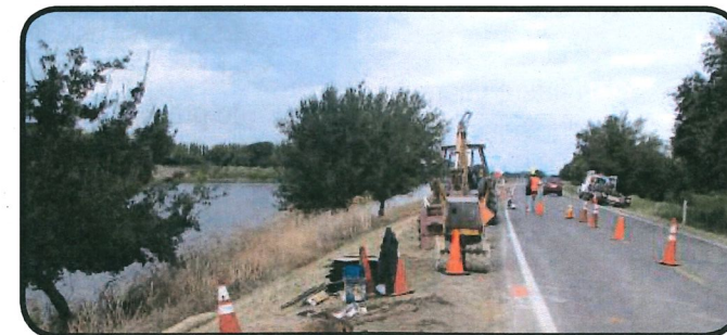
RD 551 provides repairs to levies and foundations to maintain and improve flood and drainage control systems.
